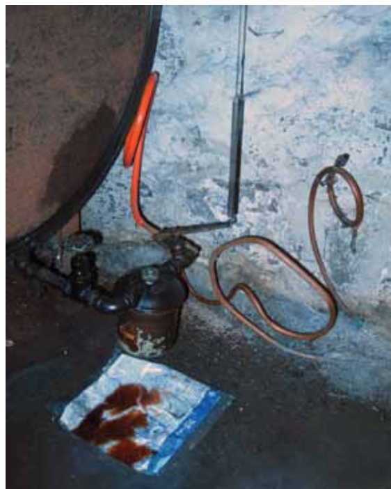
Older systems must have their uncoated lines upgraded at an average cost of $150 to as much as $600.
